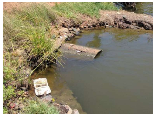
Figure 5 One of many culverts which allow water to flow in to the rural or urban area.
